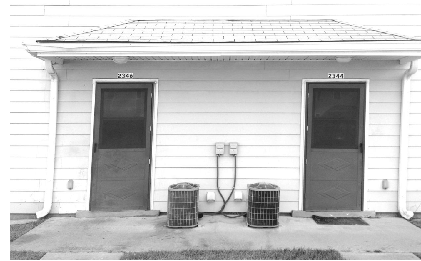
This photo shows a typical First Floor rear porch shared by two living units.
